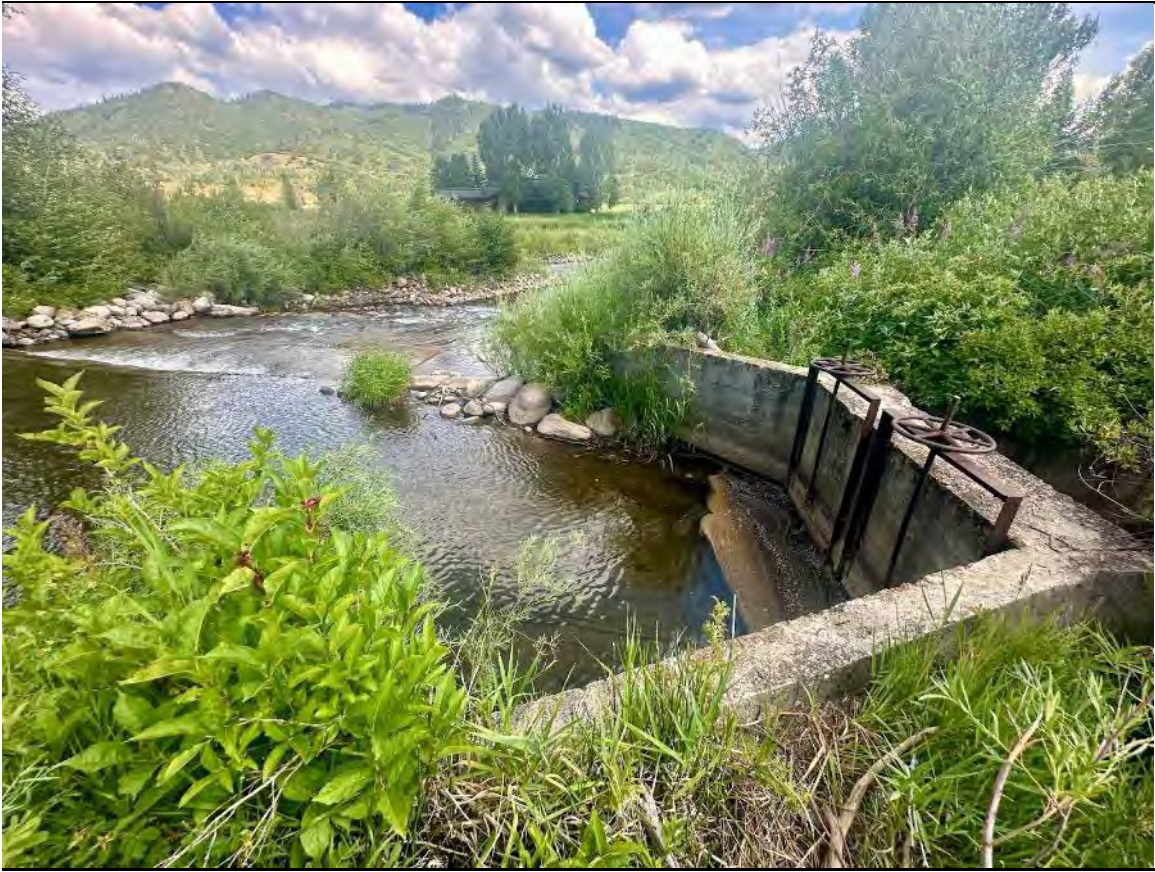
Figure A-5. Diversion structure (“push-up” dam & intake/headgate) in riverscape 9
